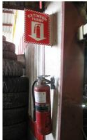
Figura 29 Extintor PQS 10 lbs.
