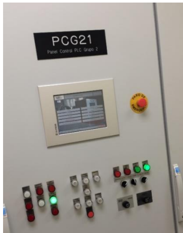
Figura 2.15 (a): Tablero de control PCG21.
