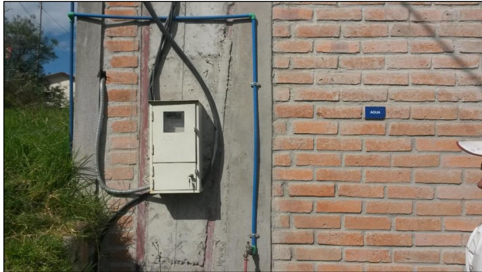
Fig. 3.3 Tablero principal (TP)
